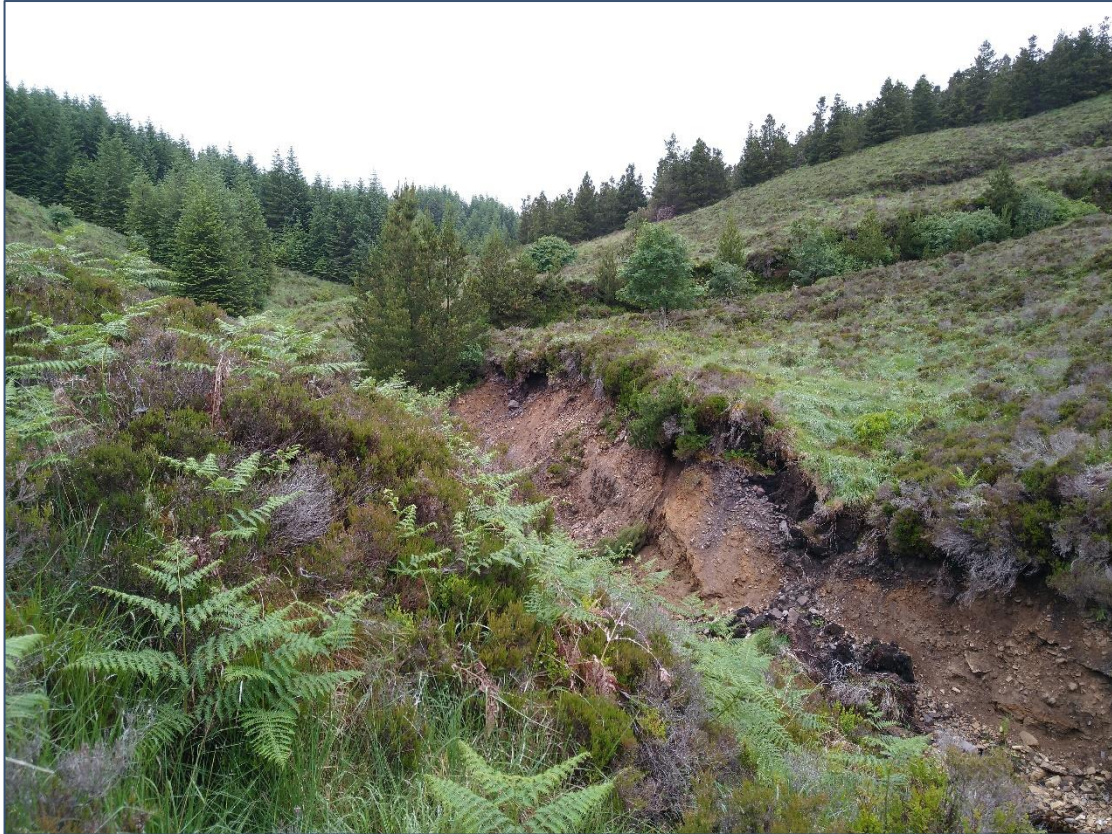
Plate 3-7 Wet Heath on either side of the river valley north-west of proposed Turbine 1
