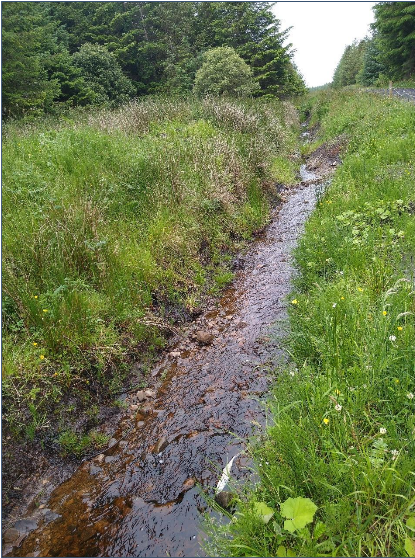
Plate 3-15 Drainage feature along the forestry road in the north of the EIAR Site Boundary.
